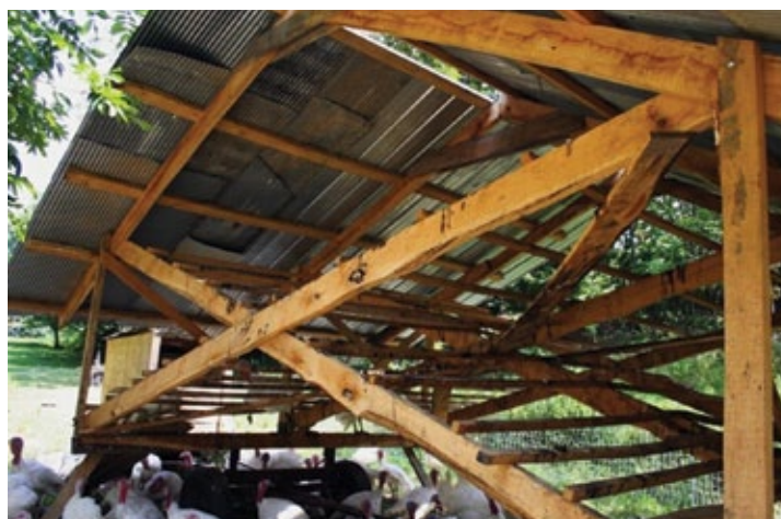
The scissor truss design of the millenium feathernet offers more protection, safety, and better use of vertical space than the old hoop house design for portable skid structures. (Photo by Rachel Salatin)
