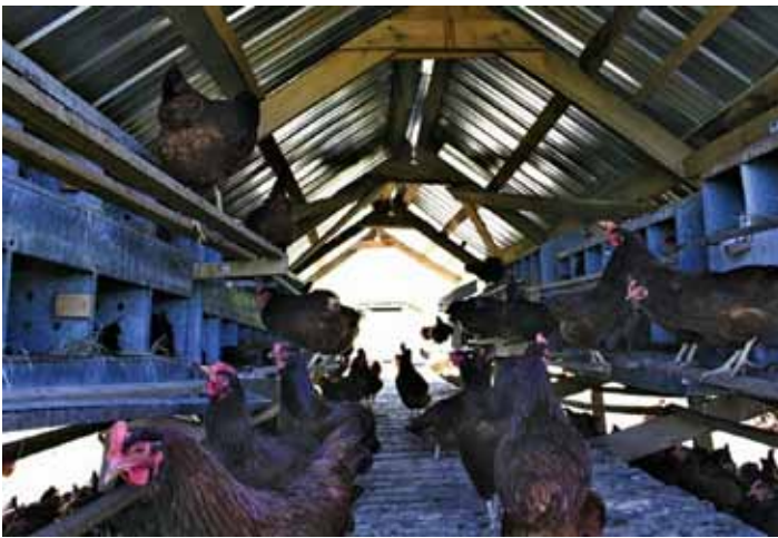
The scissor truss design of the millenium feathernet offers more protection, safety, and better use of vertical space than the old hoop house design for portable skid structures.
