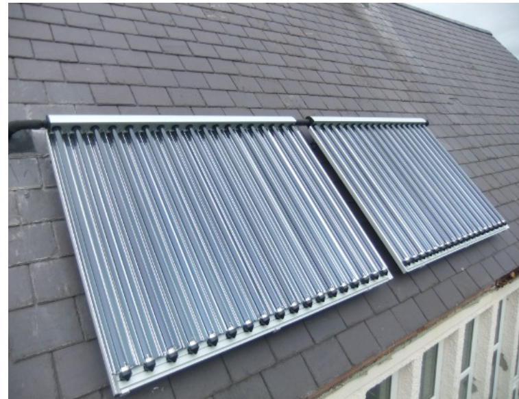
Evacuated tube solar hot water collectors
