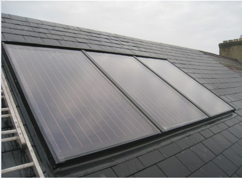
Flat-plate solar hot water collectors
